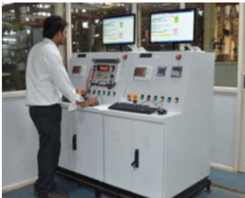
SCADA Test Facility
