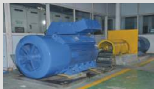
Large Motor Test Facility
